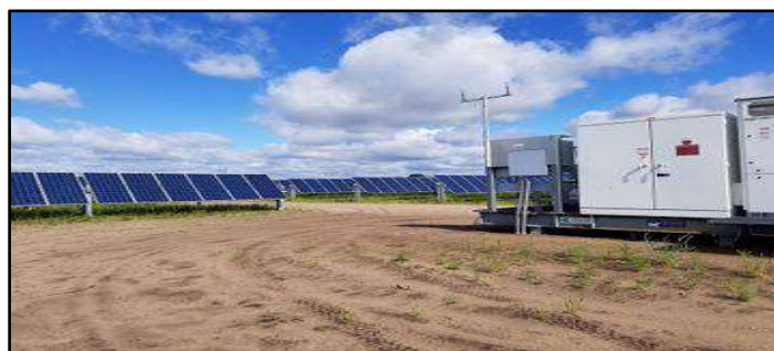
Fig-7: A photovoltaic system comprised of a solar panel cell, inverter and other electrical device.
